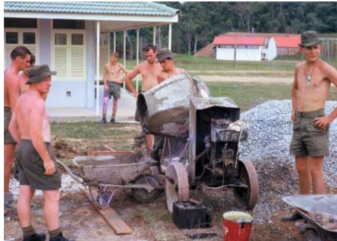
Pouring concrete for the volleyball court, the Troop's first task after arrival. The assault course and 25-yard range are in the background.
