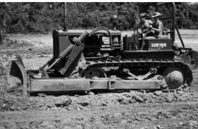
Spr Dave Wood accompanied by Spr Ian Tibbles on a Fowler light dozer beginning preliminary work on the helicopter test area adjacent to the 11 Sqn area.
